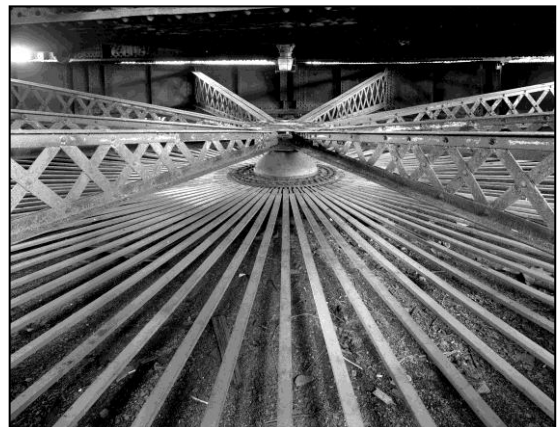
Interior of the pivot structure, showing flat-bar arms connected to the rollers and lattice girders radiating out from the center guide pin enclosure.
